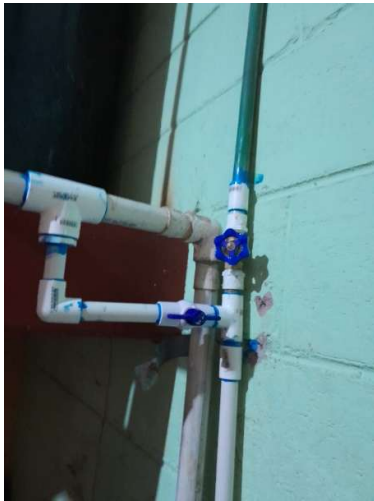
Water bypass, allowing running water for the community.
